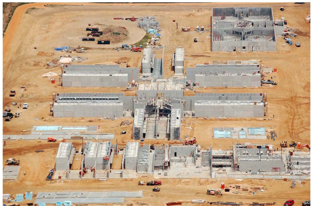
BLACKWATER RIVER CORRECTIONAL FACILITY July 27, 2009 Segregation/Support, H1, H2 & H5 Viewed Looking East
